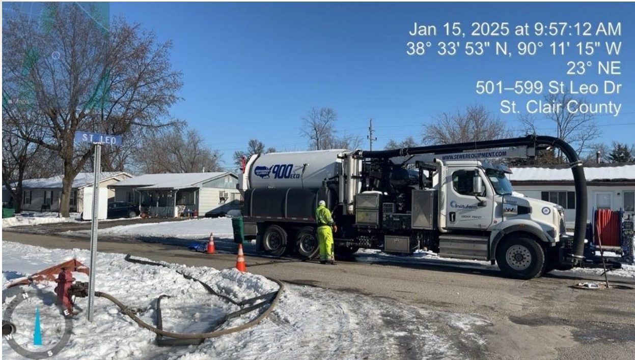
Cleaning Efforts w/ vacuum Truck
